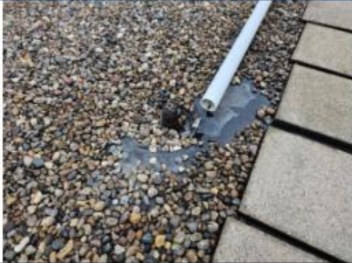
Ballast in drain
