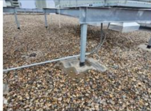
Insufficient pipe boots
