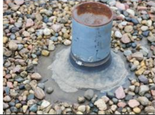
Insufficient pipe boots
